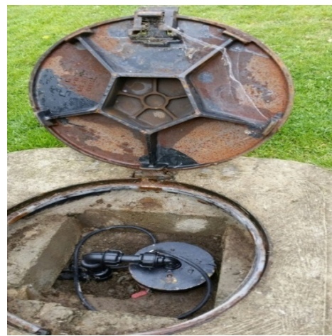
Figure 2: a borehole fully capped and sealed
